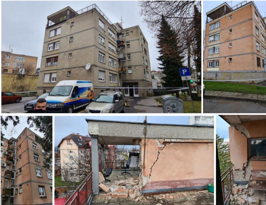
Fig. 23 Damage to multi-storey residential buildings in Zaprešić, located more than 60 km from the epicenter (CCEE 2022)
