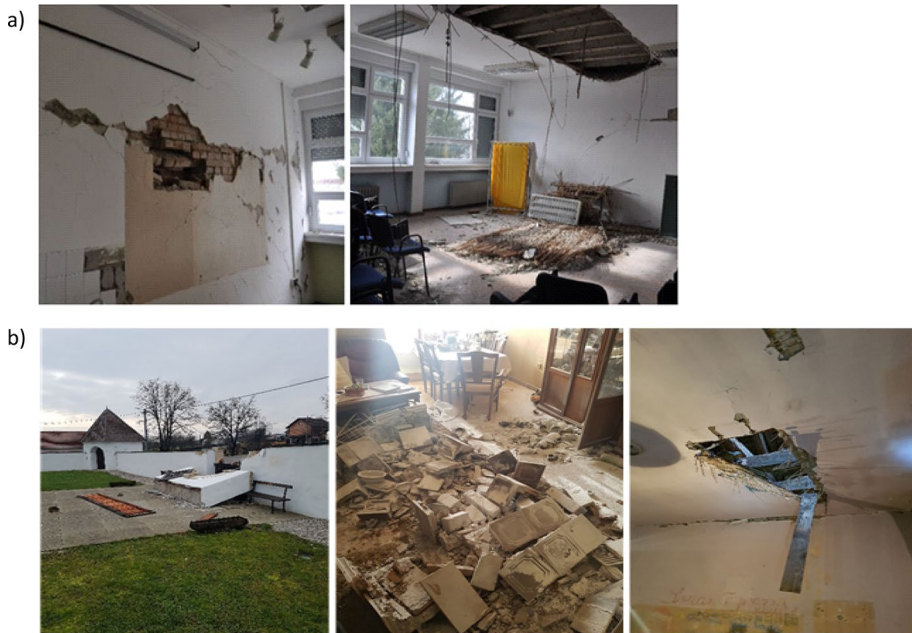
Fig. 26 Damage to non-structural elements: a failure of partition walls and plaster detachment, b toppling of the outer wall, toppling of the heavy tile stove, and hole in the floor structure due to chimney collapse (CCEE 2022)
