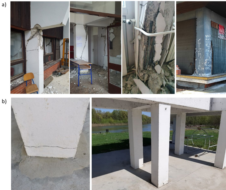
Fig. 24 Typical damage to RC building: a brittle fractures and b bending cracks in columns (CCEE 2022)
