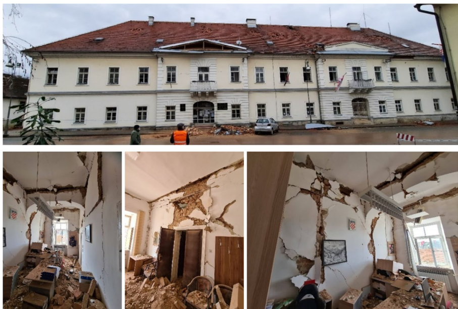
Fig. 12 Damage to buildings in the public sector, Petrinja City Hall (CCEE 2022)
