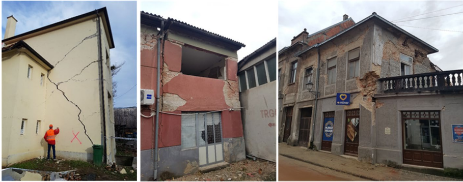
Fig. 18 Typical damage: In-plane wall failures and pounding effect (CCEE 2022)
