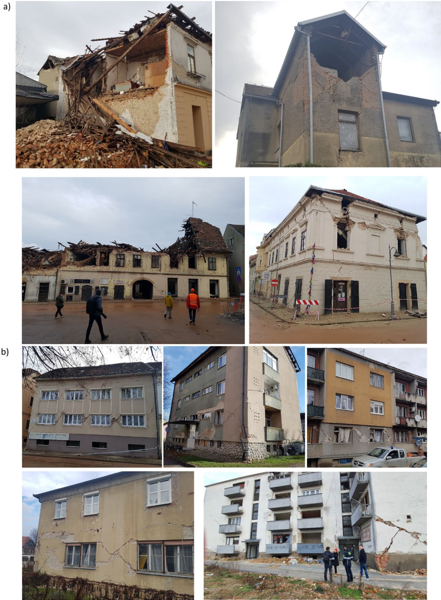
Fig. 17 Damage to unreinforced masonry buildings: a out-of-plane failure mechanisms, b in-plane failure mechanisms (CCEE 2022)
