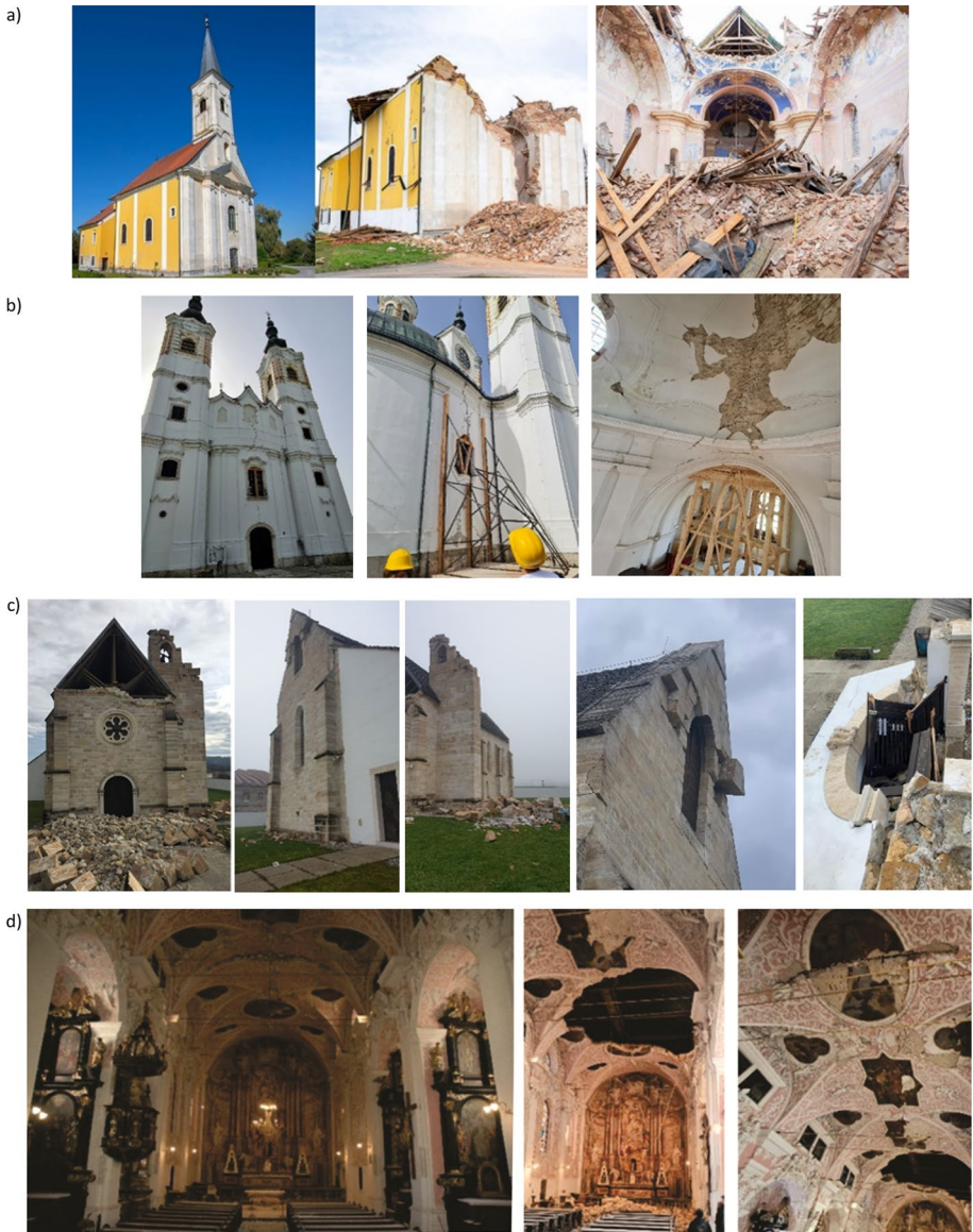
Fig. 14 Damage to sacral buildings: a Church of St. Nicholas and St. Vid in Žažina, b Church of St. Mary Magdalene in Sela, c Church of the Assumption of the Virgin Mary in Gora, and d Church of St. Catherine in Zagreb after Zagreb earthquake (left) and after Petrinja earthquake (center and right) (photos: courtesy of Sisak archdiocese 2021; CCEE 2022; and Martina Vujanović, 2022)
