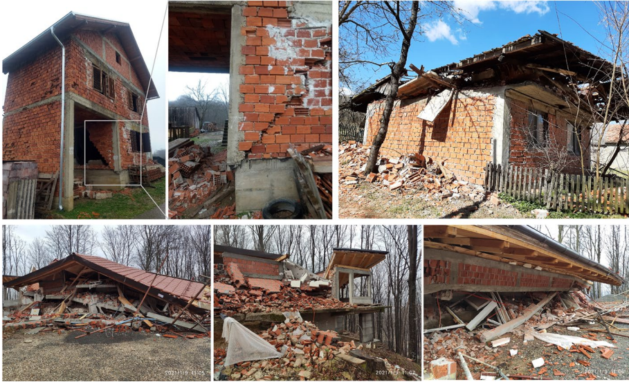
Fig. 20 Damage to (partially) confined masonry with significant structural deficiencies family houses (CCEE 2022)
