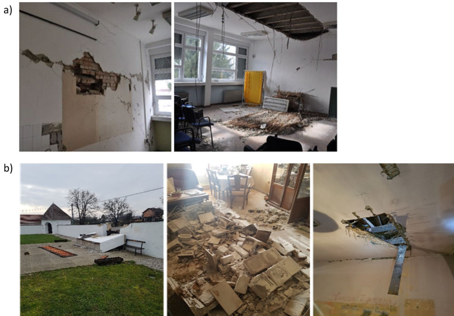
Fig. 26 Damage to non-structural elements: a failure of partition walls and plaster detachment, b toppling of the outer wall, toppling of the heavy tile stove, and hole in the floor structure due to chimney collapse (CCEE 2022)
